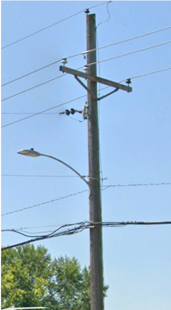
Single-phase tap pole (acceptable)
